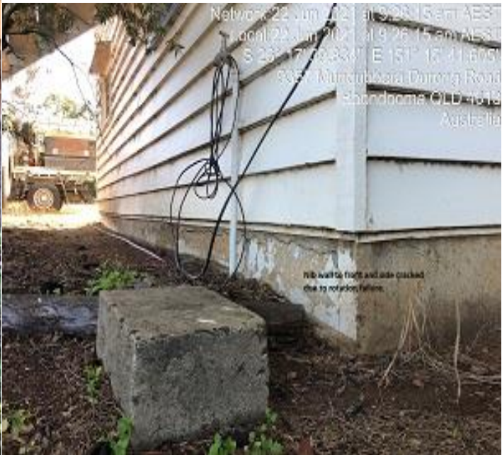
Nib wall cracked.
