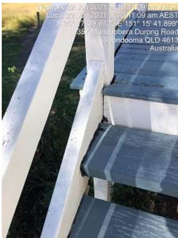
Deteriorated rear stairs.
