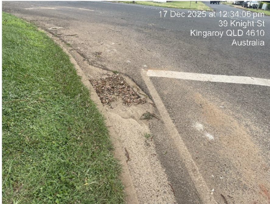
Figure 5 – Site Photo of Stormwater Inlet Pit at Corner of Kingaroy and Knight Streets.
