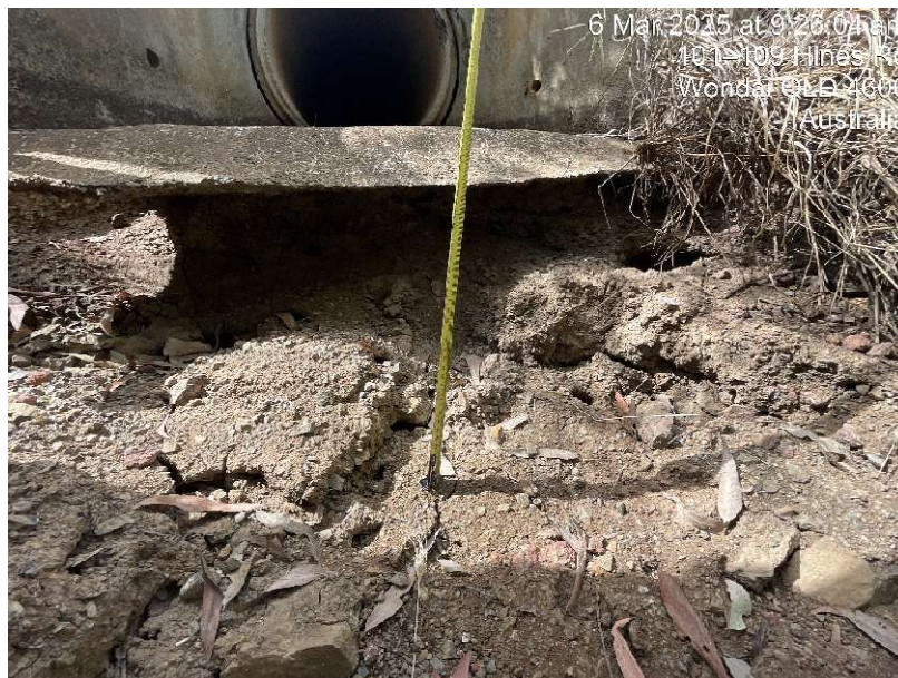
Figure 14: Erosion at concrete culvert outlet (Cnr Hustons & Hines Road).
